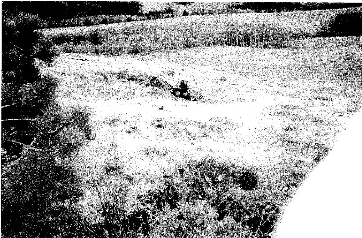
Figure 7. F7 Vein Pit II outcrop view -> S45°-50°E towards T1N trench and backhoe trenching Pit I. Vein changes to S30°E beyond Pit I.
